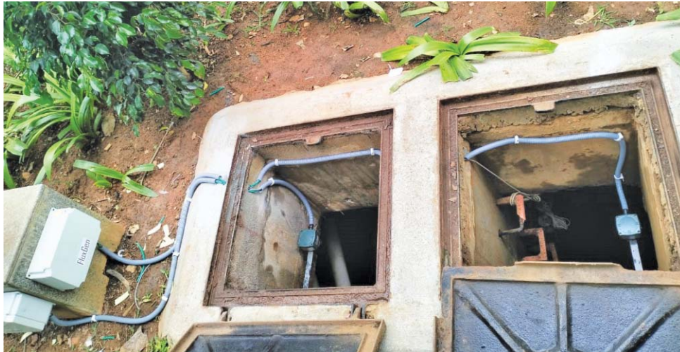
Storage tank level monitoring
