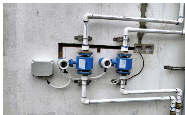
Smart water meter installation to monitor water consumption.
